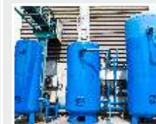
Compressed Air, N 2
