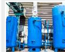
Compressed Air, N 2
