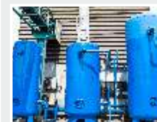
Compressed Air, N 2
