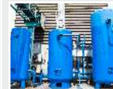
Compressed Air, N 2
