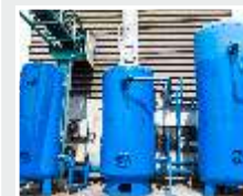
Compressed Air, N 2
